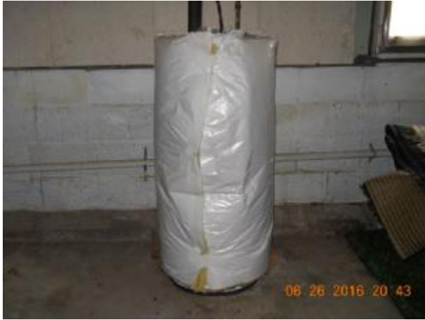
Water heater wrapped in insulation
