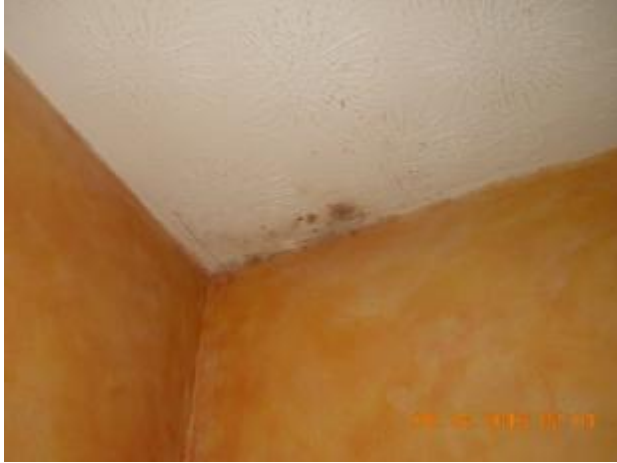
Mold in master bedroom
