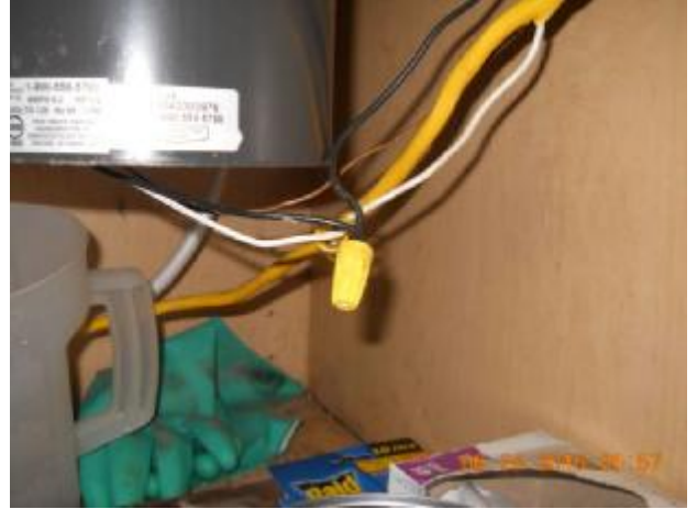
Wiring to disposal
