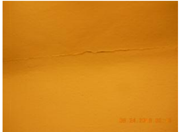
Settlement cracks on ceiling
