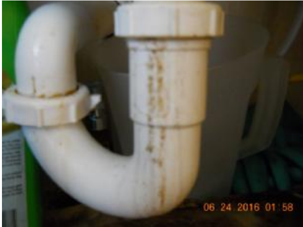
Previous leak under kitchen sink
