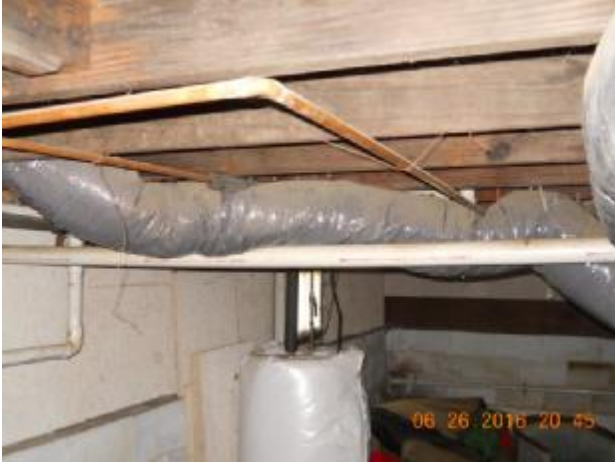
Furnace exhaust sloping down
