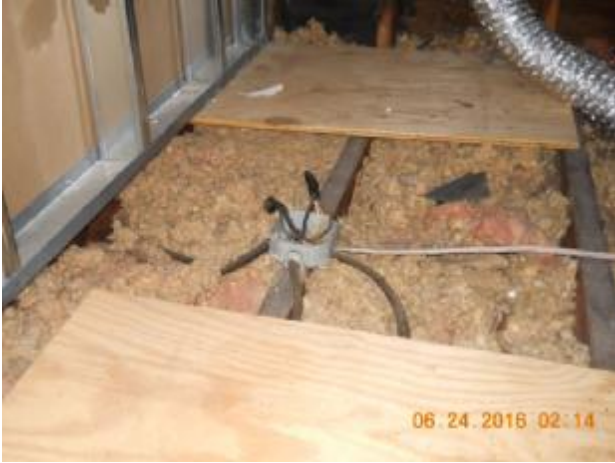
Open junction box
