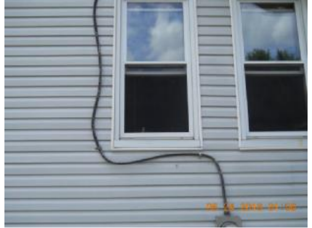
Service drop wire sheathing is deteriorating
