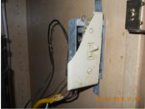
Broken cover plate
