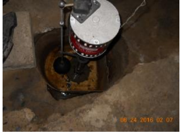
Sump pump open
