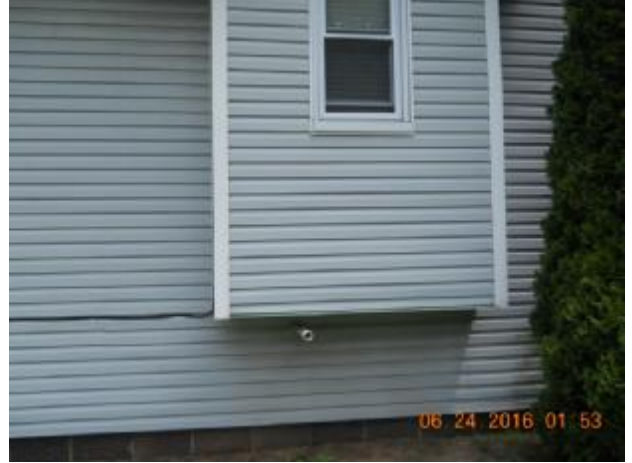
Vent below window and no screen
