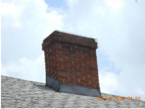
No rain cap on chimney
